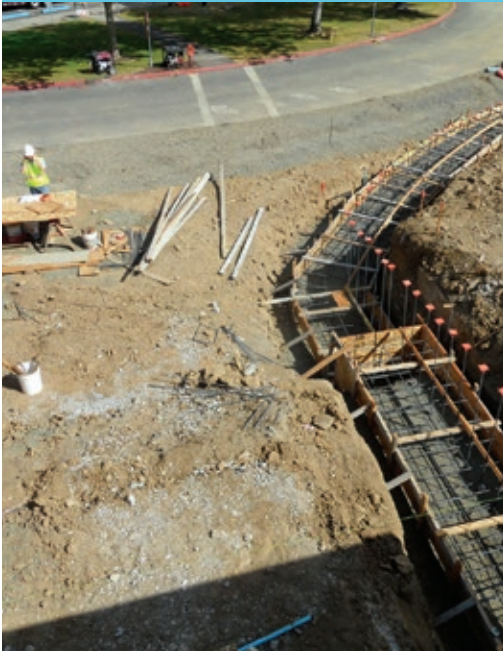
Construction of an ADA parking lot at the Howard M. Terpenning Recreation Complex
