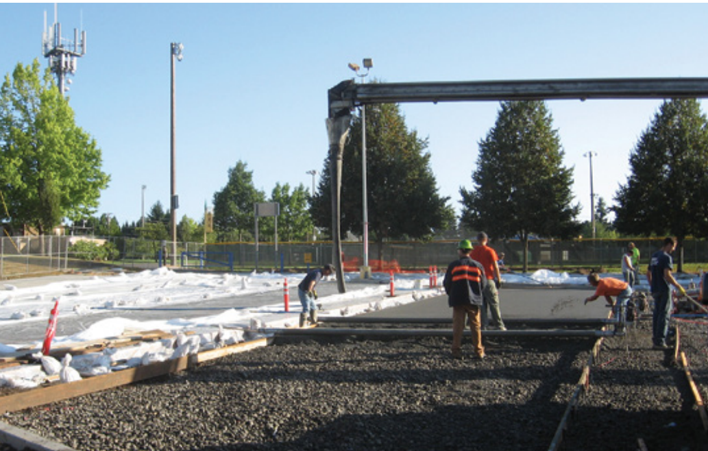
A new pervious concrete parking lot is installed at Sunset Swim Center. The environmentally friendly surface reduces stormwater runoff.
