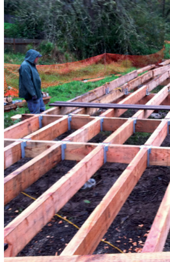
This boardwalk, part of a project connecting the Waterhouse Trail to the Rock Creek Trail, is another example of bond funds being used to increase recreational opportunities for the public.
