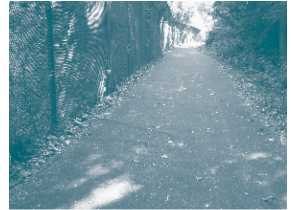
Asphalt surface being uplifted by tree roots on Fanno Creek Trail
