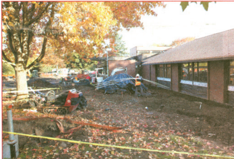
CHANGING VIEW — Seniors exercising in a workout room, top, at the Elsie Stuhr Center can keep tabs on construction workers' progress as they work on the much-anticipated expansion of the popular center at 5550 S.W. Hall Blvd.
